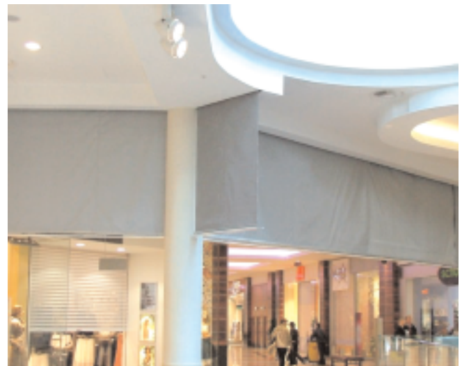
Coopers Smoke curtains with overlapping rollers with widths of 225m have been fitted to Dubai International Airport
